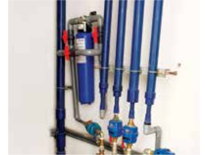
Condominium / Apartment Installation
