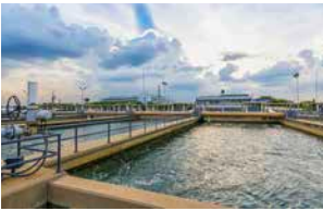
Collecting and retaining basins
