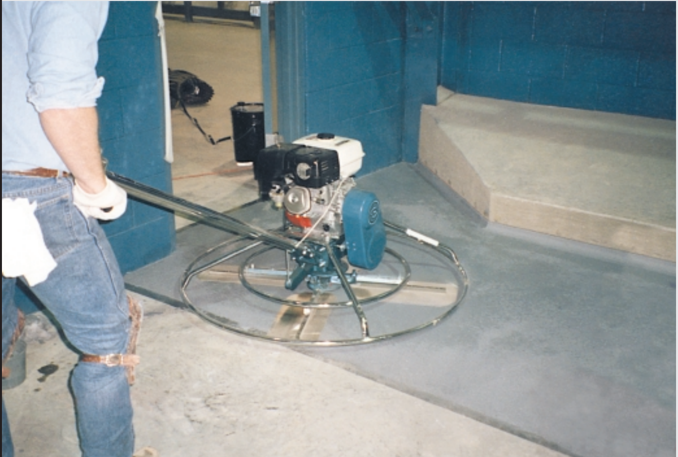
Sauereisen monolithic flooring conforms to USDA requirements.
