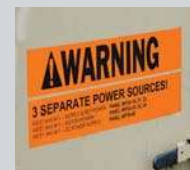
Equipment & Panel Labeling
