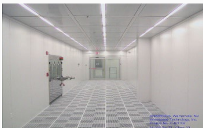
CLASS 100 CLEAN ROOM
