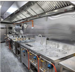
ELECTRIC & GAS EQUIPMENT
