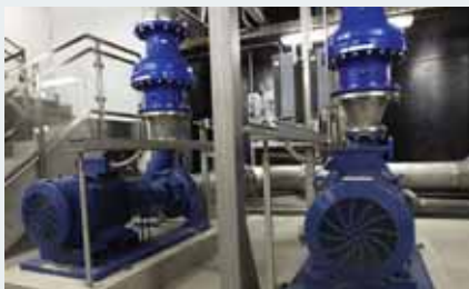
Water supply, Wertheim, Germany Raw water from deep wells is treated in a three stage process. VLT® AQUA Drives make it possible to balance these three processes to maximise treatment performance.
