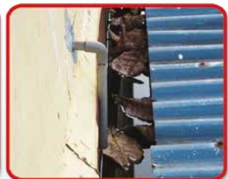
Clogged rain gutter
