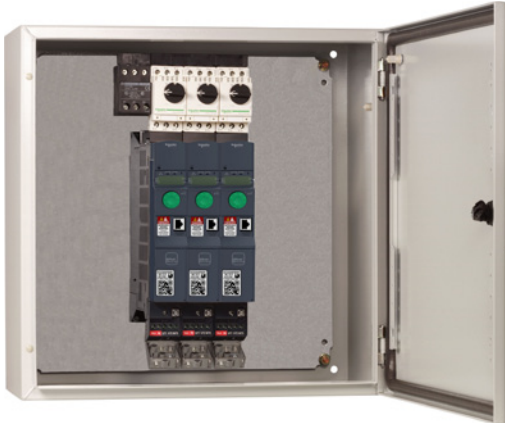
Example of GV2/ATV320 direct mounting in an enclosure: GV2L circuit-breakers + GV2454 and GV2G05 accessories + ATV320U15N4B drives
