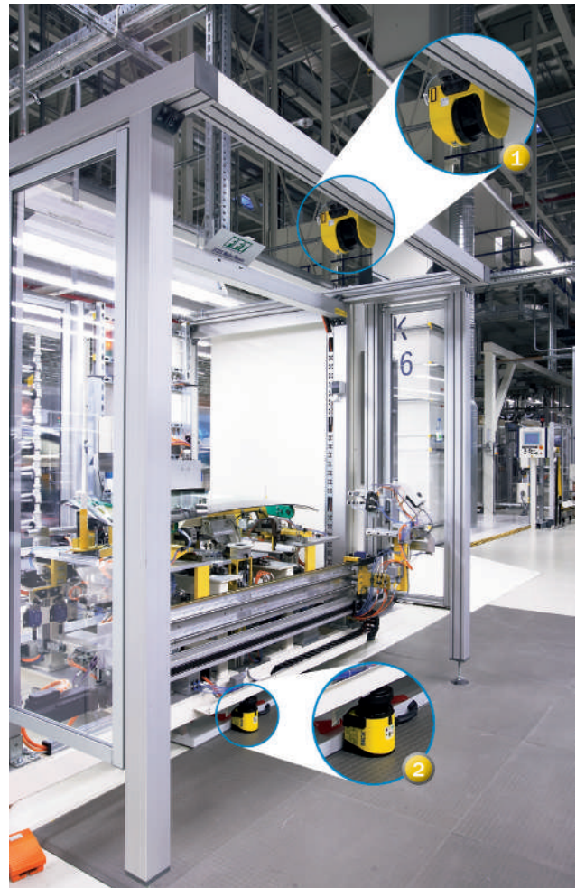
Figure 79: Safety laser scanner on a machining center as safety function pos. 1, initiating a stop and safety function pos. 2, preventing start (presence detection)
