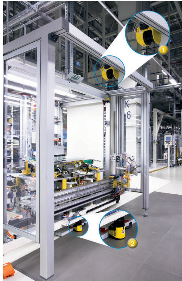
Figure 79: Safety laser scanner on a machining center as safety function pos. 1, initiating a stop and safety function pos. 2, preventing start (presence detection)
