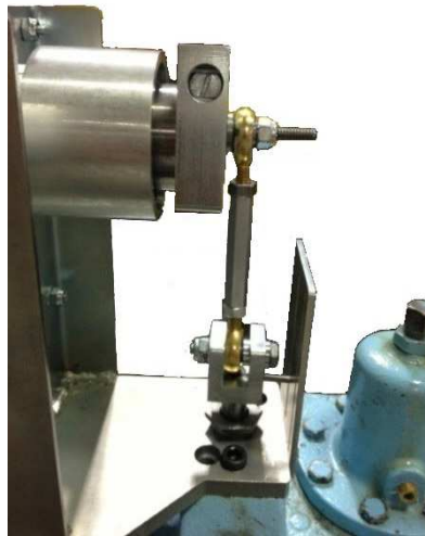
Figure 10: Bracket Mounted to Fuel Oil Controller
