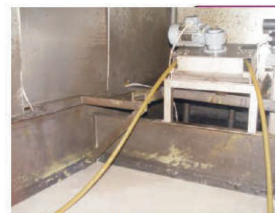
Oil skimmer model W40 at waste water tank
