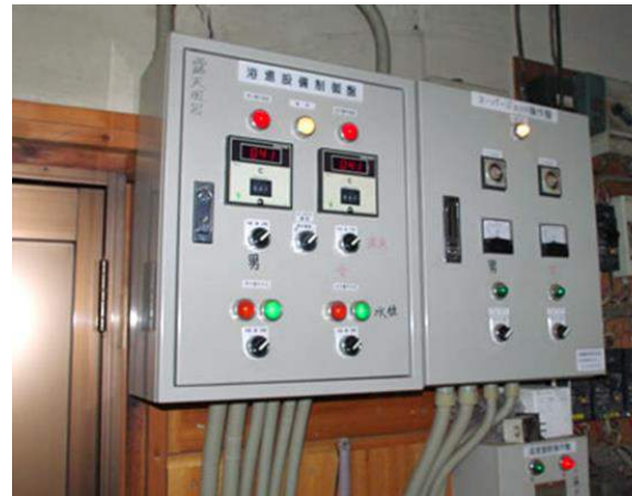
Also can find the other company's meter.
