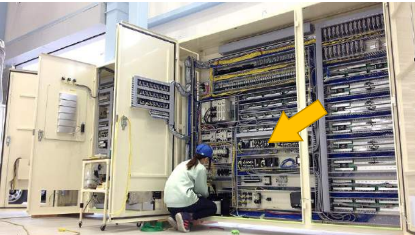
2) Just open the door of control panel. Signal converter is installed inside of control panel .
