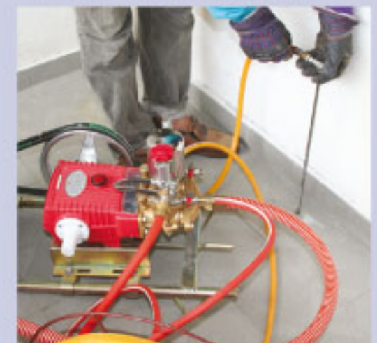
Premise 200 SC injected through slab. Each hole is filled with 5 liters solution.
