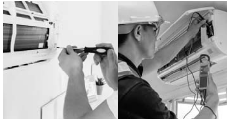
Complicated Wiring Steps Difficult Connecting
