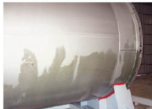
Avesta FinishOne™ Passivator 630- removes free iron (the brown staining seen on the photo).
