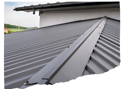
METAL, PLYWOOD, ROOFTILES
