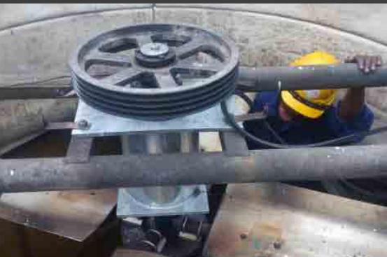
Replacing complete fan bearing assembly, pulleys for all brands of cooling tower.
