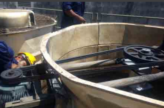
Replacement of fan belt, pulley, motor & entire drive system for all brands of cooling tower
