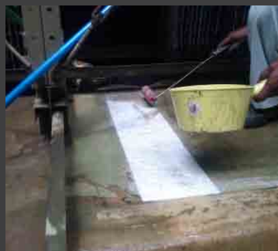
Lamination of FRP surface to repair leaks for all brands of cooling towers.
