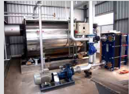
Hot water boiler for CTI test facility
