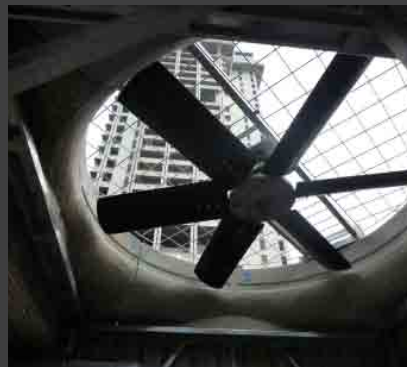
Replacement of existing cooling tower fan blades for all brands
