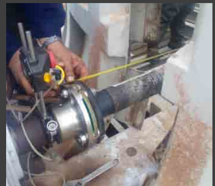
Alignment checking for gear reducer drive (shown above) and belt drive system.
