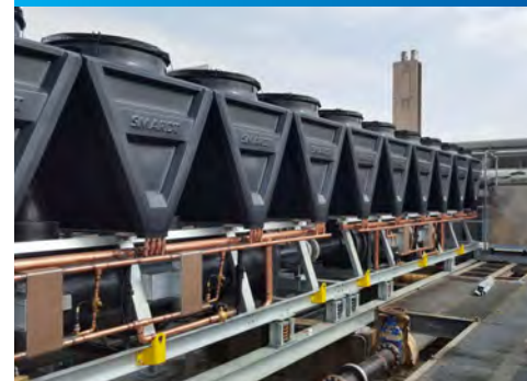
This T-Class air-cooled installation at a major hospital in Hong Kong is one of a series – specified because of lowest lifecycle costs and high reliability with unmatched redundancy.
