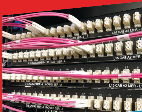
Fibre optic cabling
