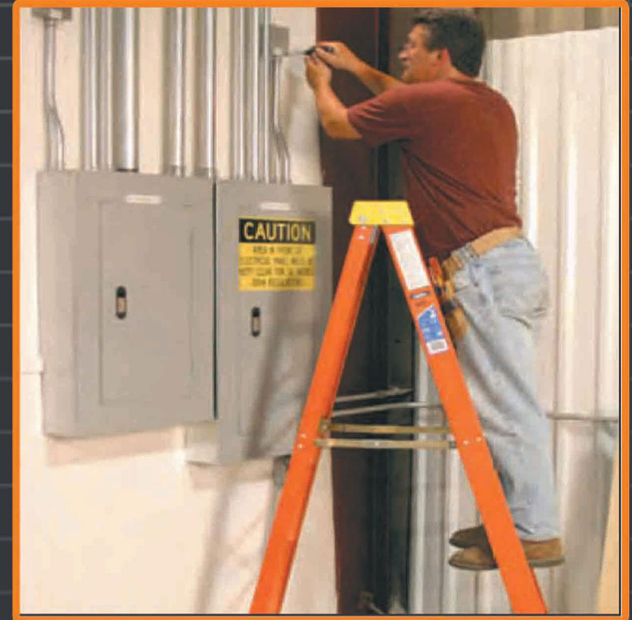
Use fiberglass ladders if there is even a remote possibility of working near electricity or overhead power lines.
