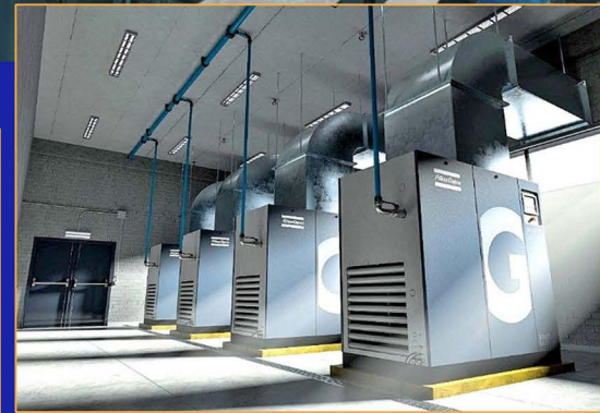
Air-con Compressor Plant
