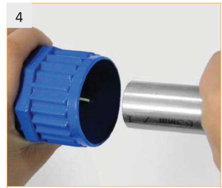
4 Lightly deburr inside and outside edge. Level up 0.3mm x 45° (0.012" x 45°) permissible.
