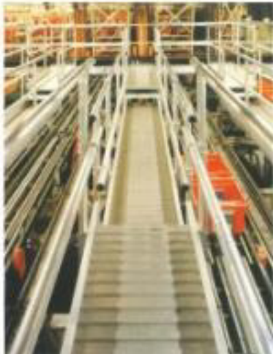
John Lewis Partnership - Access to truck parking conveyor system in warehouses.
