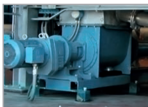
WANGEN KL-R pumps in operation
