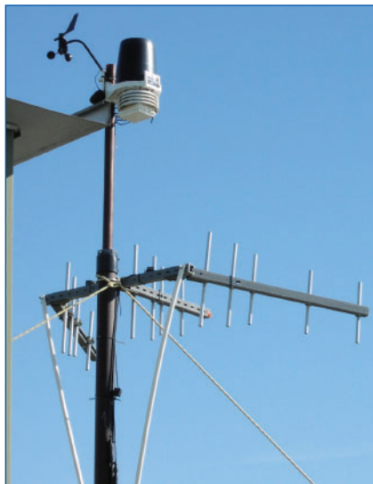
(Left) The RiverSonde antenna mast. Three 0.5-meter Yagi antennas are arranged symmetrically in a tight sector. A weather station atop the antenna mast provides wind and meteorological data.
