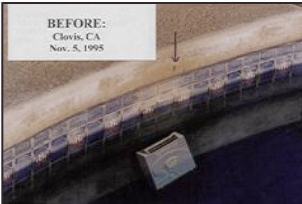
Unsightly scale deposits were a constant problem for this swimming pool in Clovis, California before the ScaleBlaster™ unit was installed.
