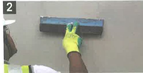
2 Smoothen surface with LiquidRender 2000(F) (0.5mm) to get a marble-white smooth finishing wall
