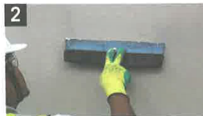
2 Smoothen surface with LiquidRender 2000(C) (1mm) to get a sandstone-white finishing wall
