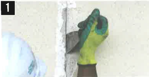
1 Chip away sides of crack to form channel and provide keying surfaces
