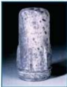
Rapid corrosion of untreated aluminium
