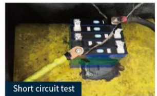
Short circuit test
