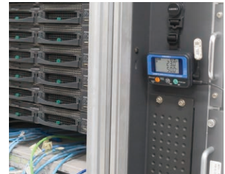
Recording temperature and humidity in a server room
