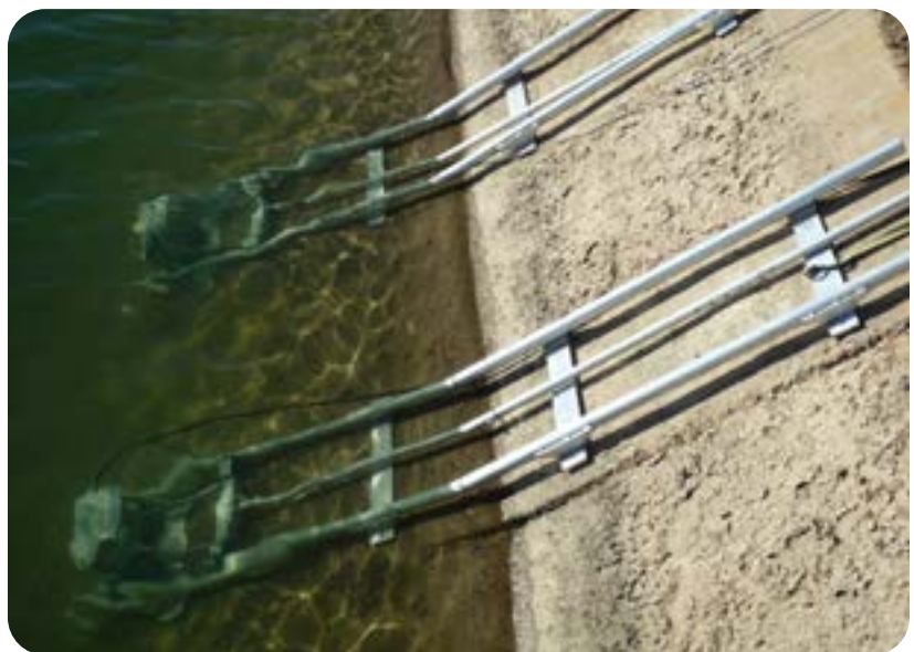
Example of a typical SonTek-SL1500 concrete lined canal installation as part of a HydroMet station.
