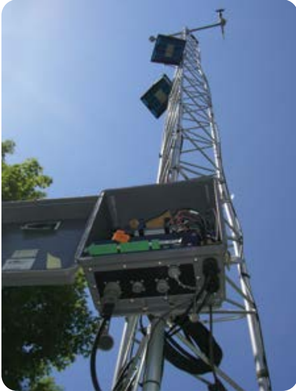
Monitoring tower containing a YSI Data Logger, and meteorological sensors
