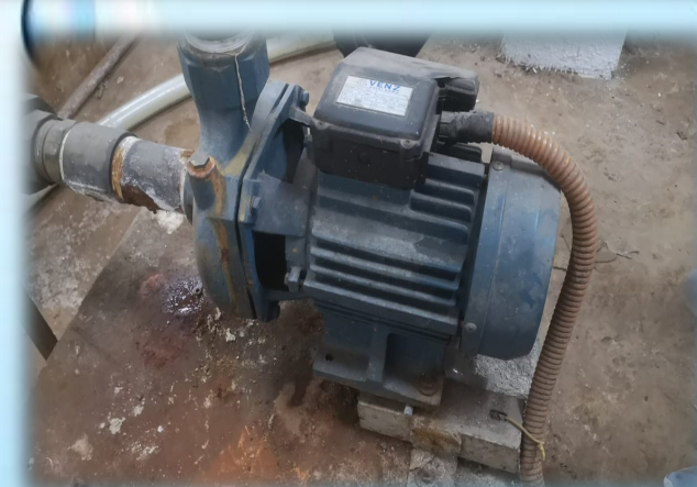
HYDRO PUMP & PANEL BOARD SYSTEM
