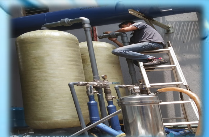
WATER FILTER SYSTEM
