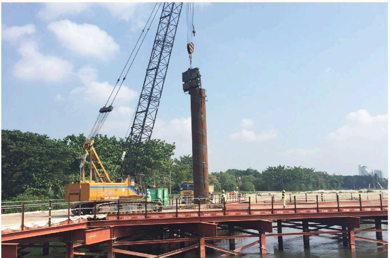
ID1500 x 16mm thk x 12m long steel casing for West Coast Highway bore piling work, Klang
