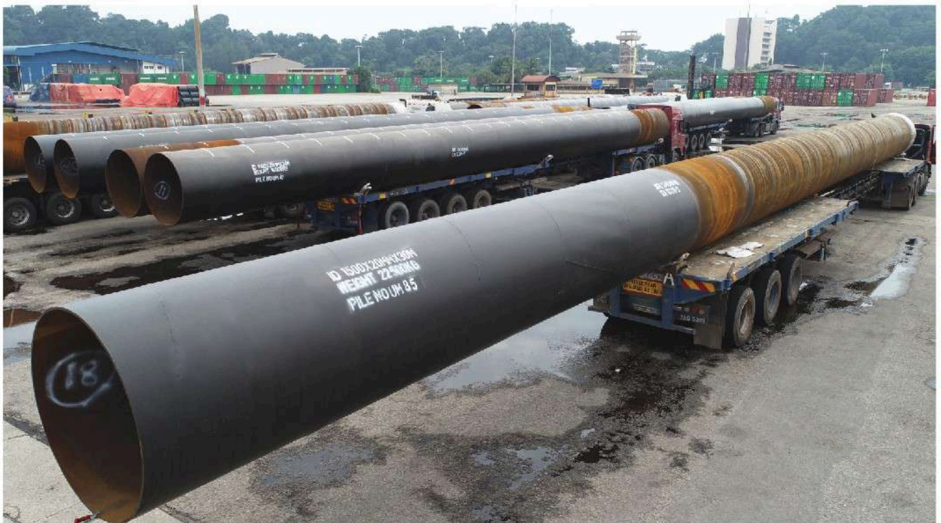
ID1500 x 20mm thk x 30m long steel casing for Pasi Road to Sibul/Tg Manis Road
