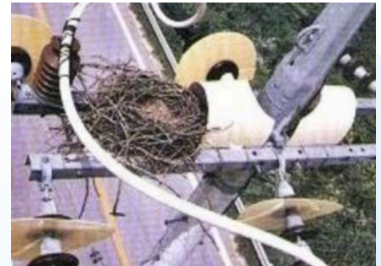
Failure of removing Nests
