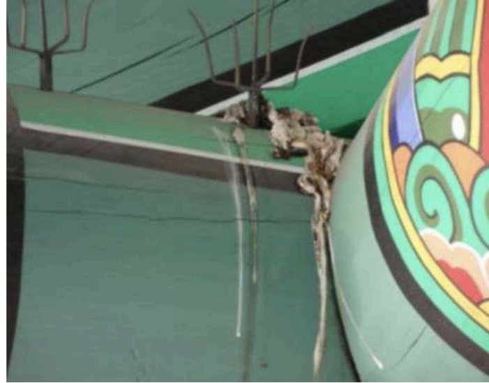
Failure of Needle Hill 1
