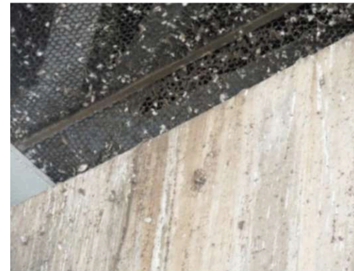
Failure of Netting 2
