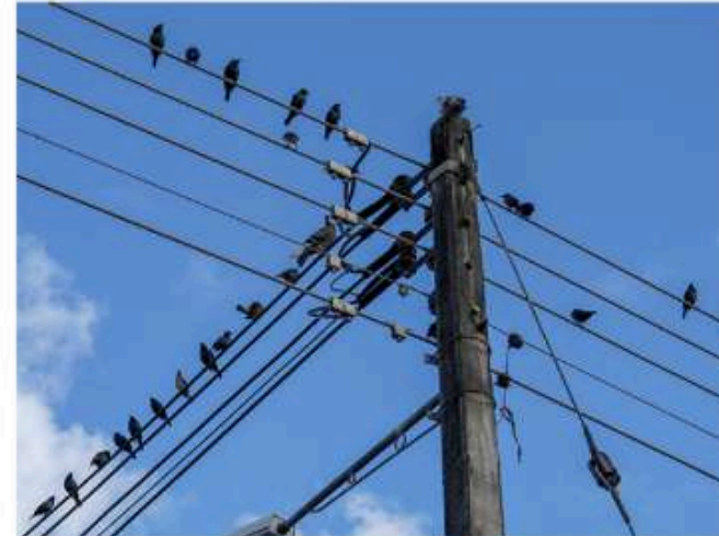
Damage caused by Crows
