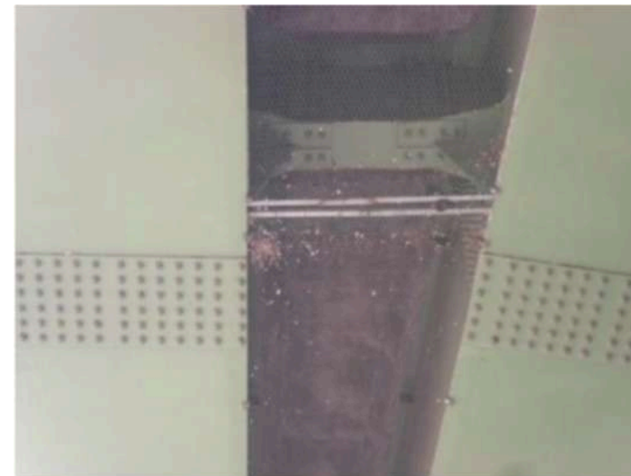
Failure of Netting 1
