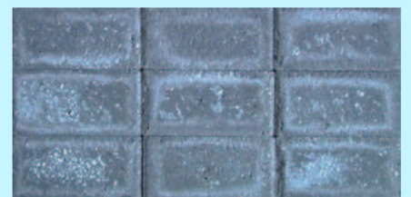
The effects of efflorescence on concrete blocks
